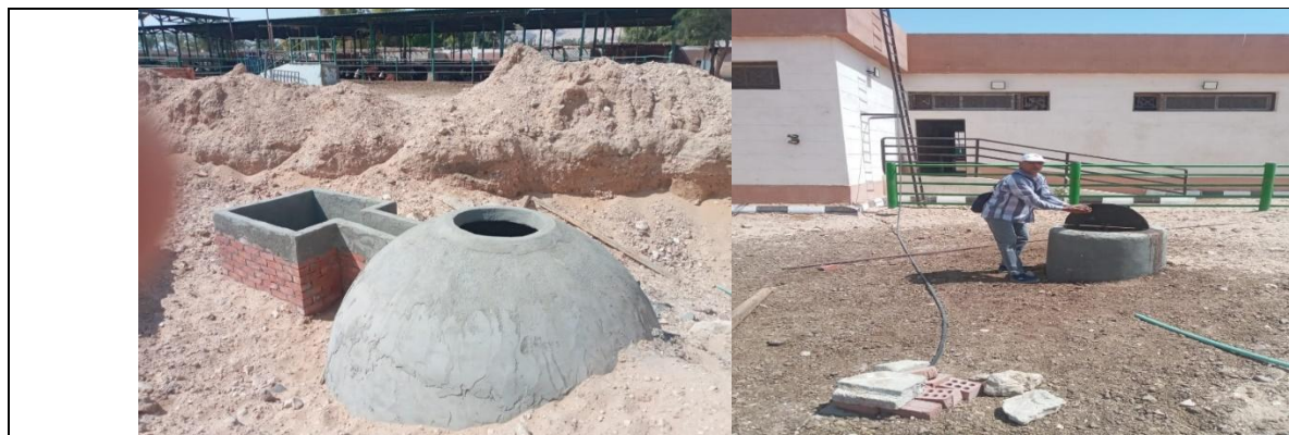
1- Building biogas generating units from organic waste (Sohag University)
